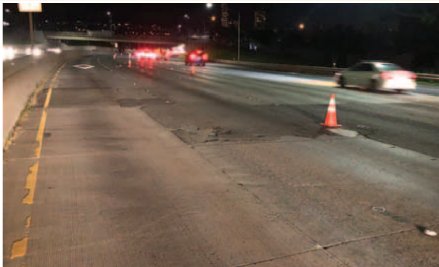
FIGURE 2 Typical site conditions before rehabilitation. (Source: Hawai'i DOT.)
