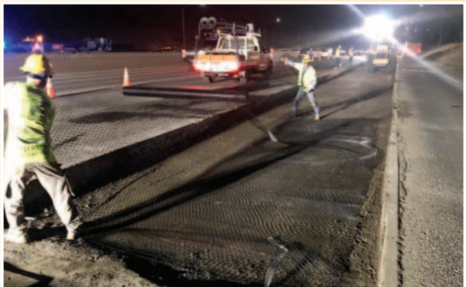
FIGURE 6 Localized installation of geogrid reinforcing in CTB for improved pavement support. (Source: Kiewit Infrastructure West Construction.)
