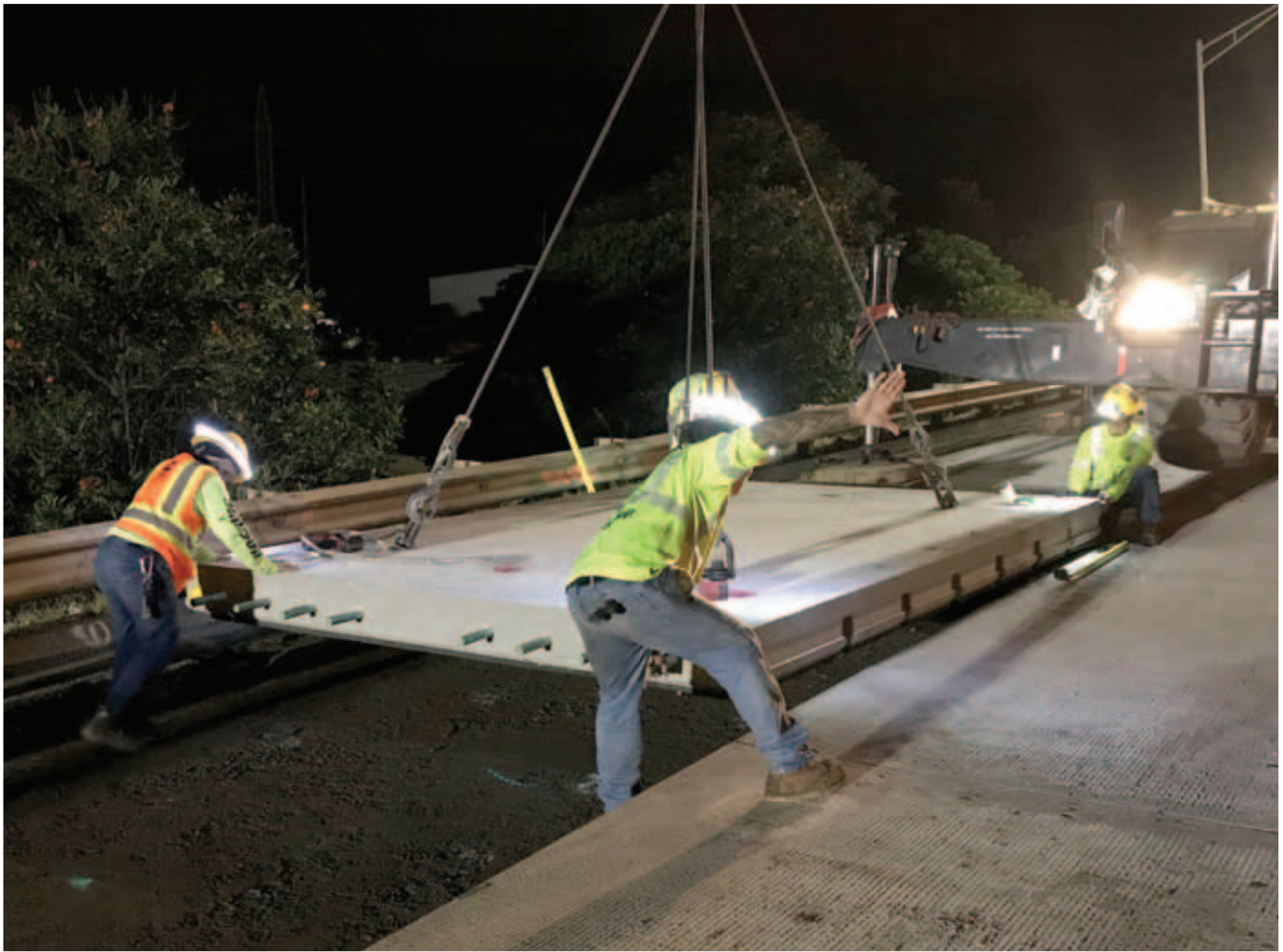
FIGURE 9 Setting precast panels in outside lane of H-1. (Source: The Fort Miller Company.)
