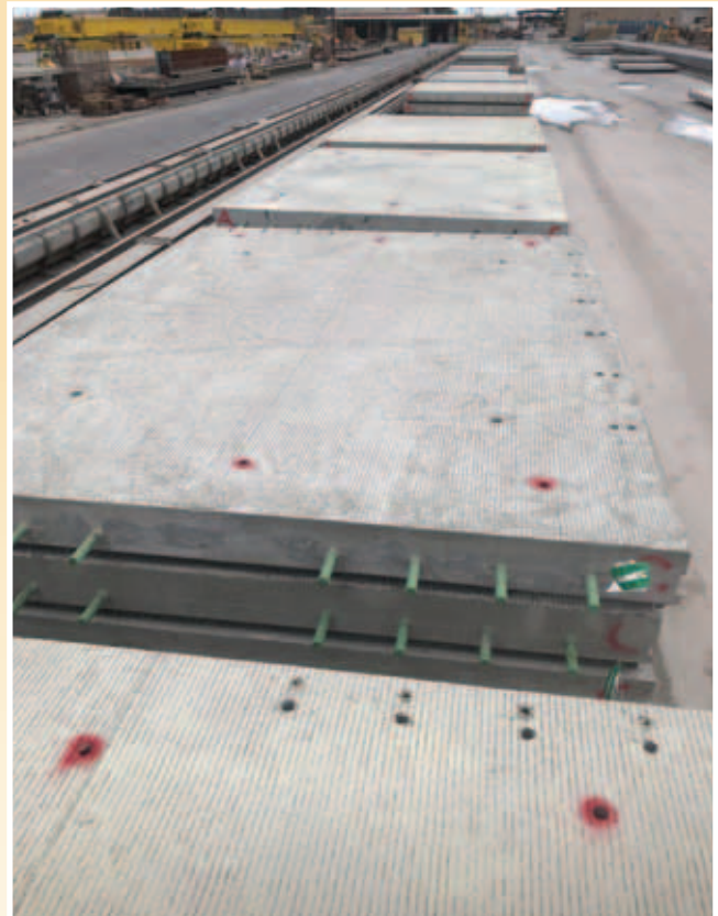
FIGURE 4 Stockpiling fabricated precast panels for H-1 project in precaster's yard. (Source: Kiewit Infrastructure West Construction.)
