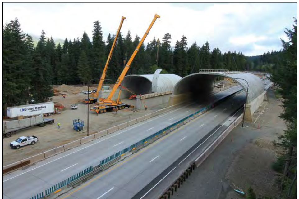
FIGURE 4 Installing a prefabricated wildlife overpass along I-90 Snoqualmie Pass East in Washington. (Source: Contech Engineered Solutions.)
