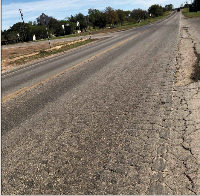
FIGURE 1 Typical fatigue cracking in asphalt pavement.
