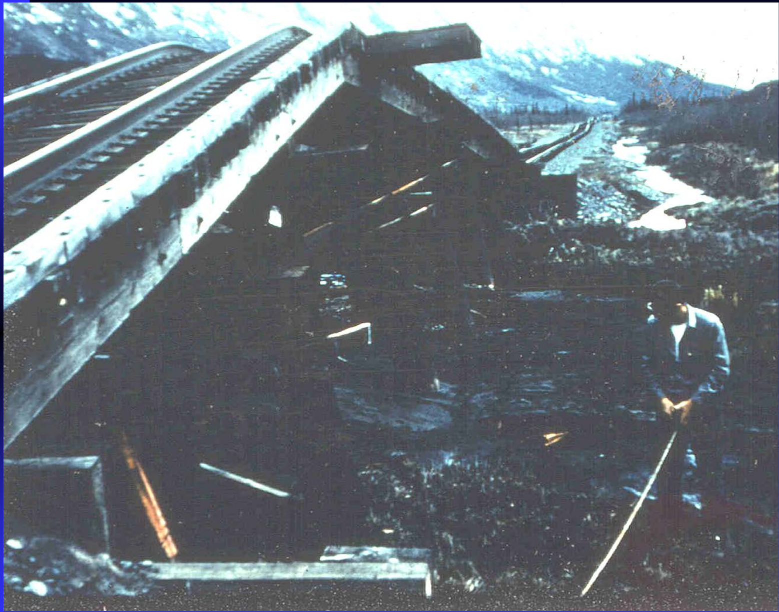
Buckled Railroad Bridge Caused by Lateral Spread During the 1964 Alaska Earthquake
