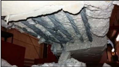
CFRP rupture Tension failure
